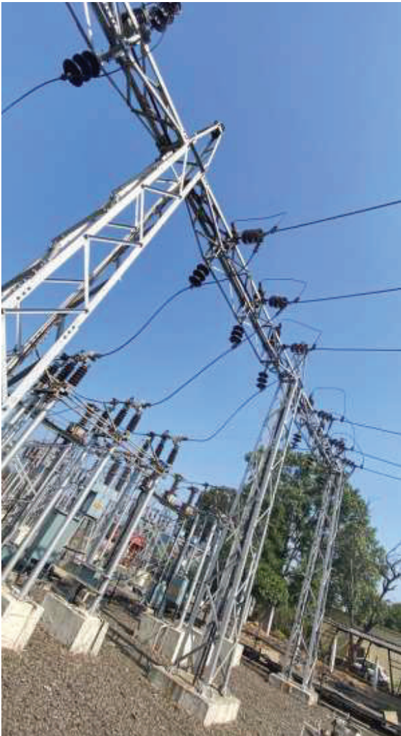
Fig. 1 : Surge Arrestors connected to separate earth pits.
