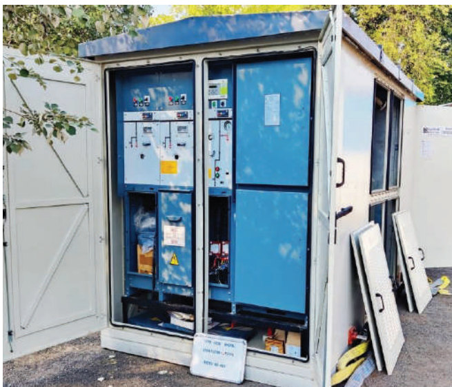
Fig. 3 : High voltage switchgear and controlgear compartment
