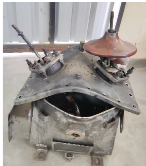
Fig. 1 : Current transformer's physical condition after fault.
