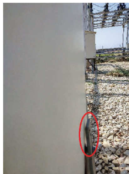
Fig. 6 : Improper earthing connection to the panel.
