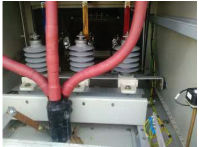
Fig. 3 : Surge arrestors connected through insulated busing.
